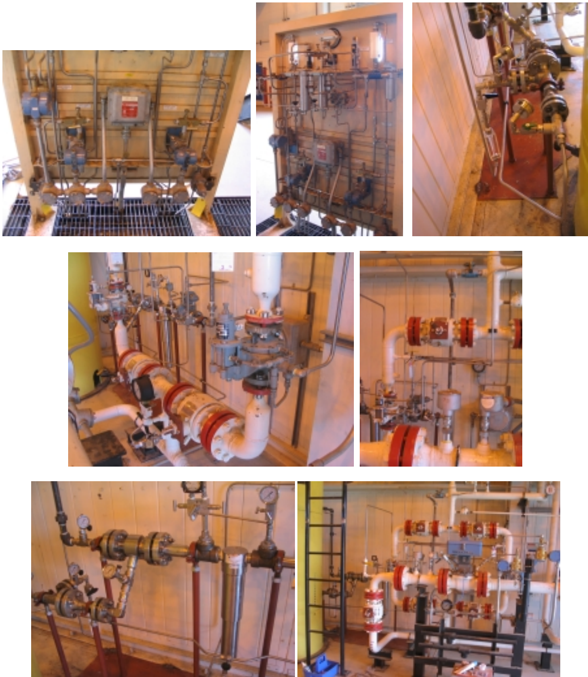
Figure 13: Photos of the Two-Stage Supersonic Ejector Skid Connected to the Fuel Gas System at a 24 MW Gas Turbine Unit.
