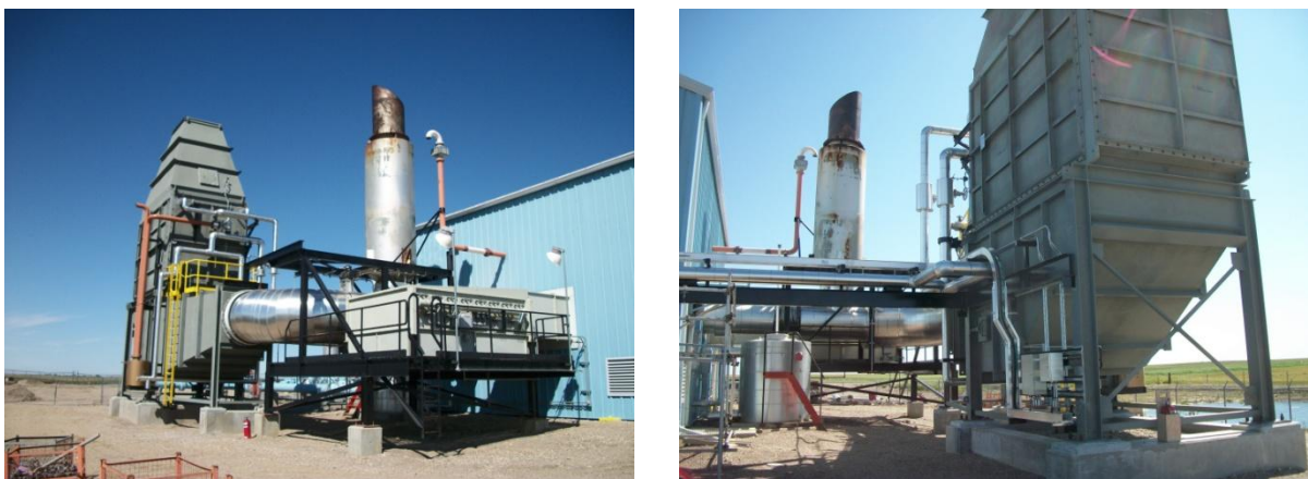
Figure 2: Waste Heat Recovery Oil Heater and Bypass Stack at the TransGas Rosetown Compressor Station
