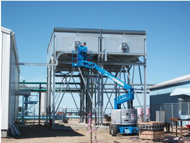
Figure 6: The glycol/water-to-air coolers for the TransGas Rosetown ORC Plant
