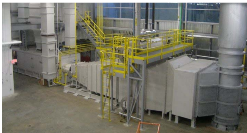
Figure 10: Refurbished LHSC Co-Generation Plant Installed (HRSG)
