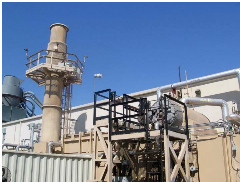
Figure 6: Original Co-Generation Unit (HRSG)
