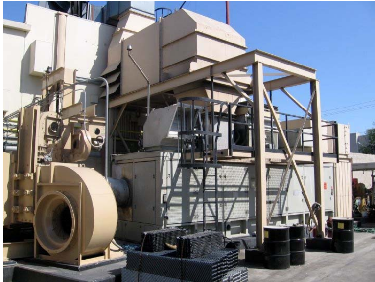
Figure 5: Original Co-Generation Unit (Gas Turbine Enclosure)
