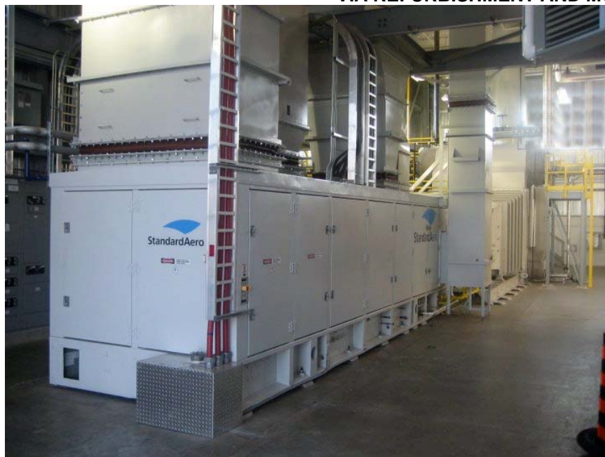
Figure 9: Refurbished LHSC Co-Generation Plant Installed (Gas Turbine Enclosure)
