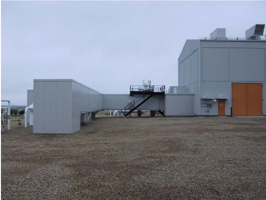
Figure 2: Fully enclosed above-grade gas piping and valve.
