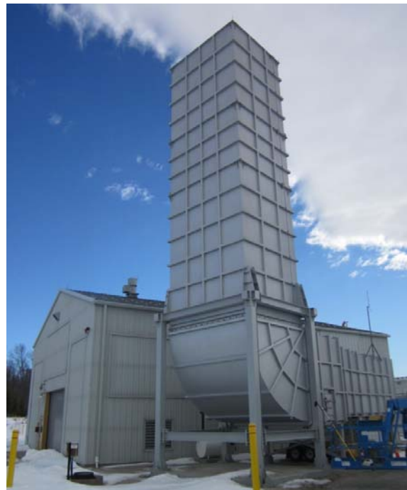
Figure 1: An industrial gas turbine combustion exhaust silencer.
