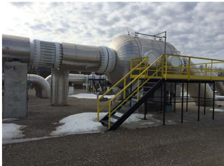
Figure 3: Above-grade gas piping with acoustical lagging applied.
