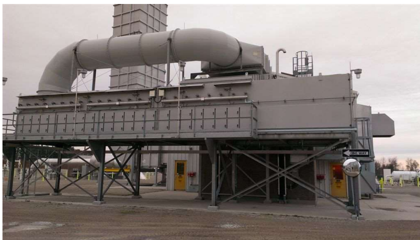
2x side by side RB211 gas turbines
