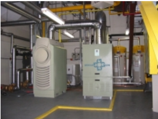
Capstone Microturbine & Heat Recovery, Minto
