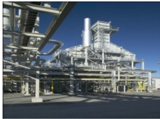
Steam System at GTAA Cogen Plant
