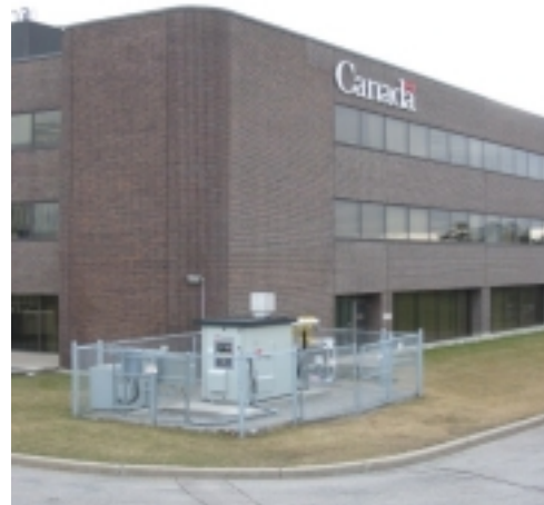
Heath Canada Microturbine CHP
