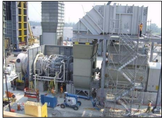
TCPL Portlands, GE Gas Turbines (OPA)
